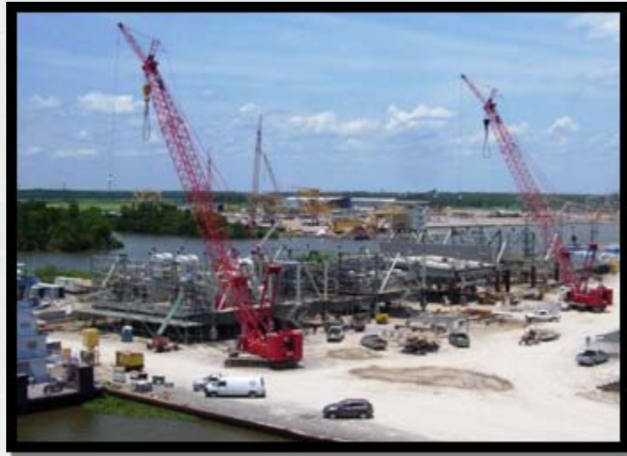
ENI Alaskan Utility Module (est. 3,600 tons)
