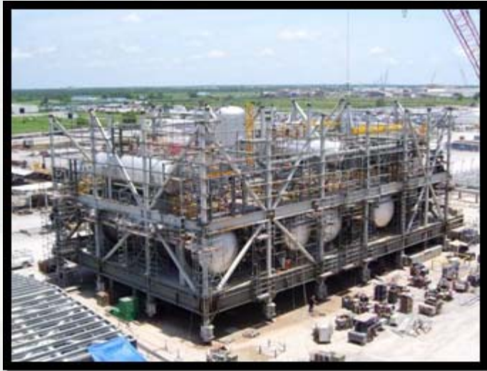
ENI Alaskan Process Module (est. 3,800 tons)
